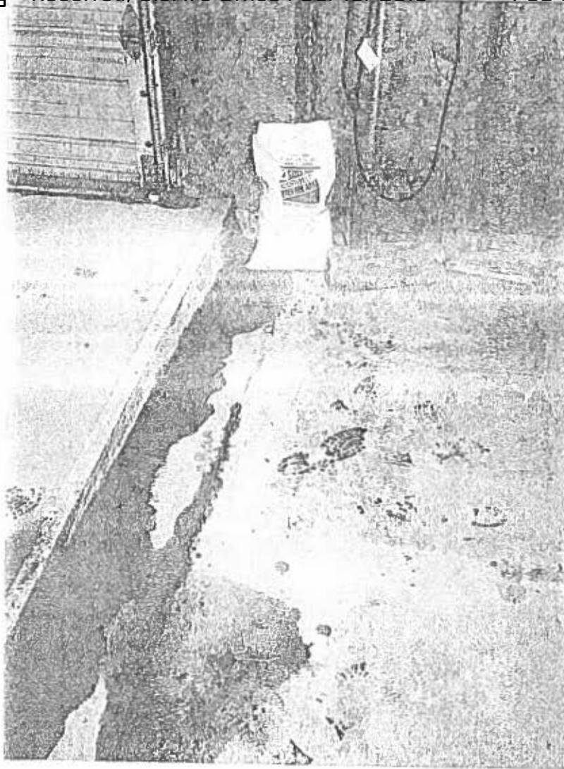
Ware house 48' x 88' Ramp at North door showing incline from ground level into warehouse 43-033-08
